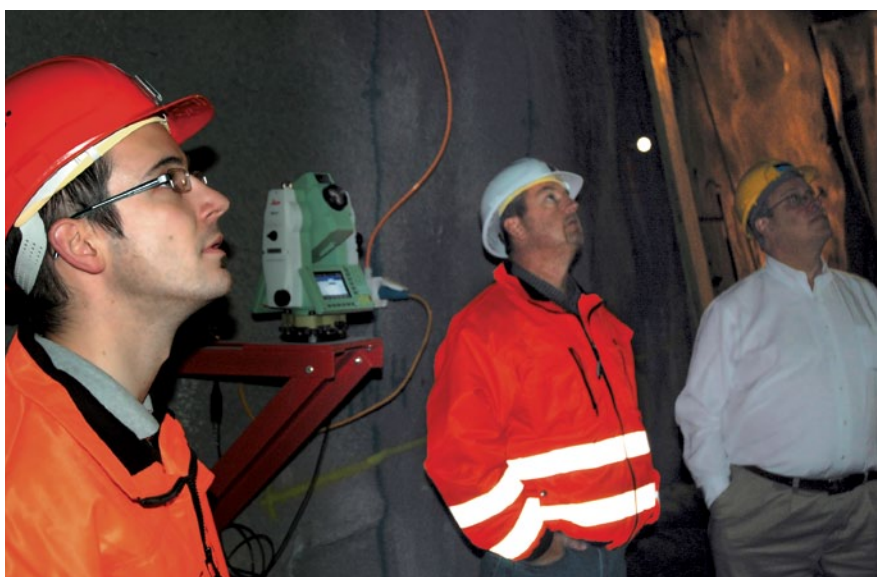
L-R Tunnel Surveying Engineer Oliver Schneider, North America Manager Brian Daniel and editor Marc Cheves watch as the TPS 1200+ is automatically guided by TMS Profile to quickly gather tunnel profiles.
