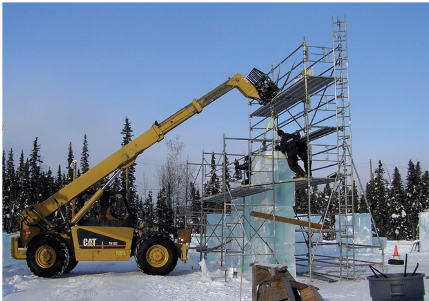
Modern tools like metal scaffolding and a long reach forklift sped up the construction process, resulting in a finished product in just 11 days.
